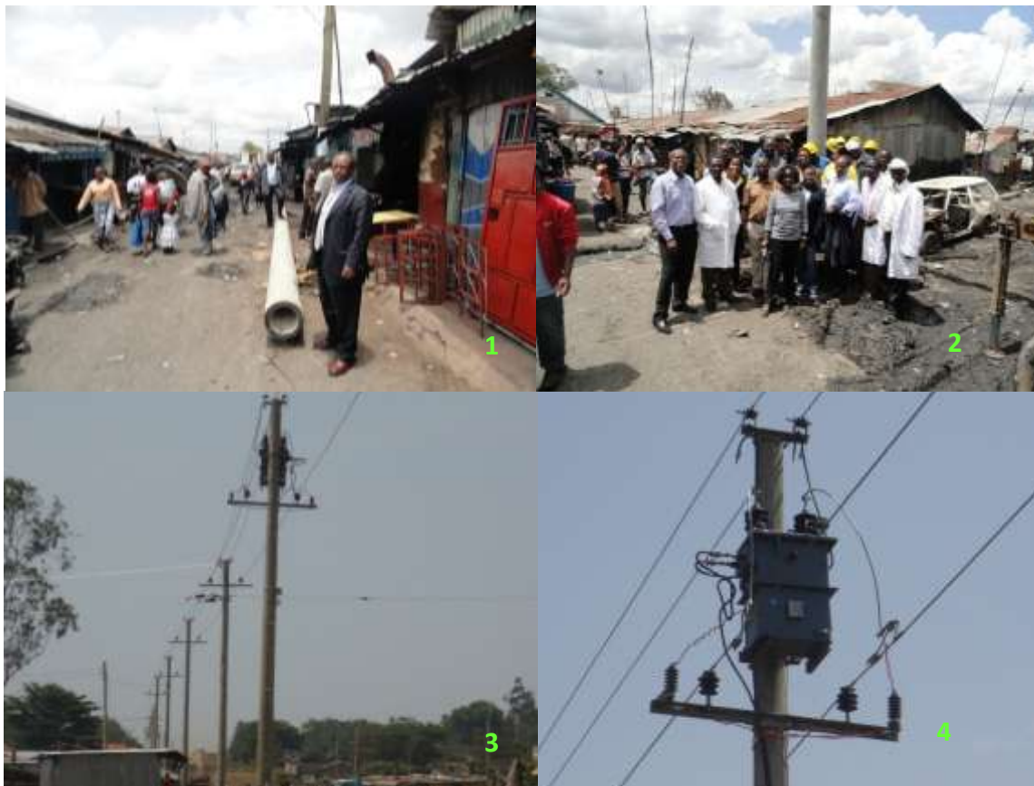
Photo 1: Delivery of the electricity poles in Mukuru slums in Nairobi. Photo 2: KPLC staff poses in front of the first pole erected in one of the slums in Nairobi. Photo 3: A typical power structure in the slums; Photo: 4: Power transformer.
