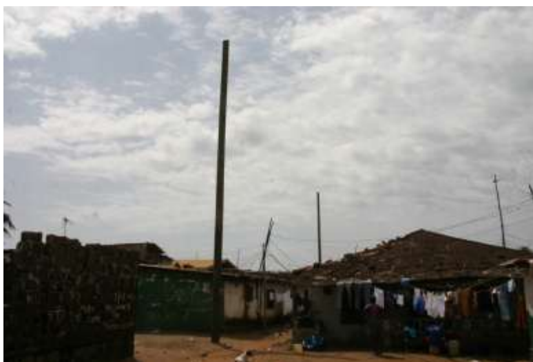
Illegally connected electricity in one of the slums in Monrovia
