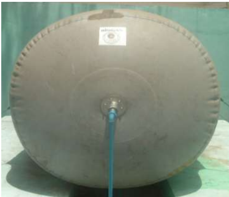
Biogas collection and storage balloon at the CUC. The gas is used in cooking and heating purposes in the laboratories
