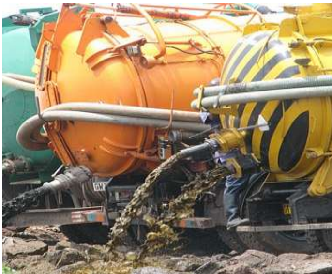
Exhausters were used to handle wastes from the ablution block at an extra cost to the hospital
