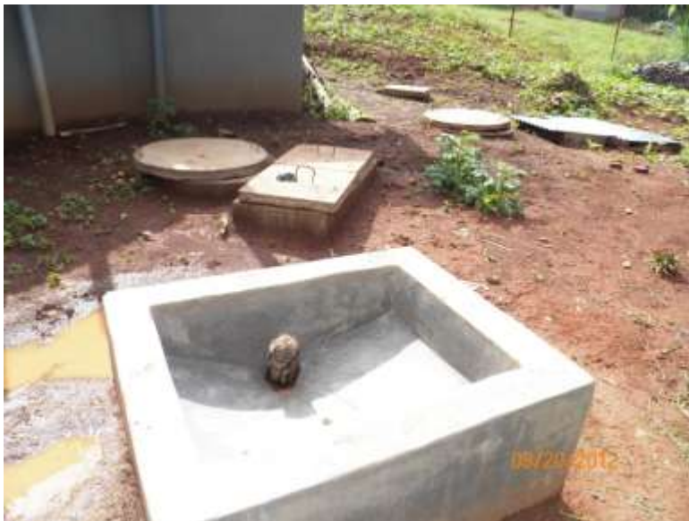
An inlet into a biogas digester
