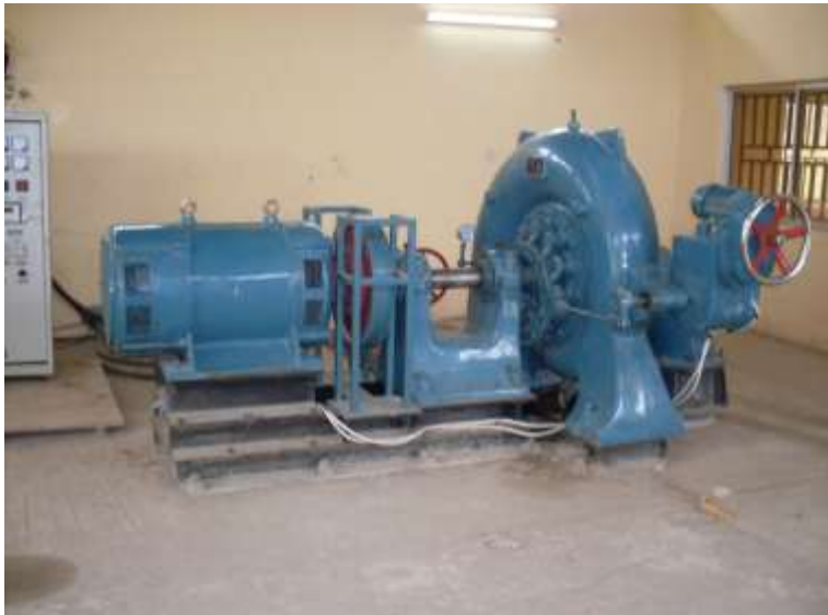
Completed Waya Project Showing the installed Francis turbine
