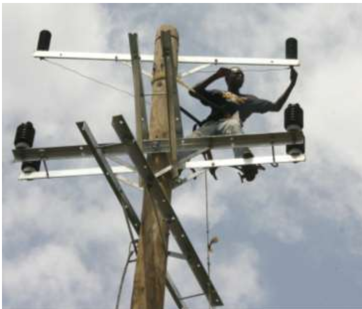
An electricity technician in the process of getting the low income households in Monrovia connected to the national grid
