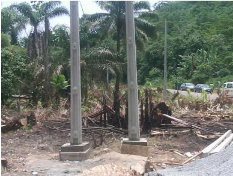
Power Evacuation poles
